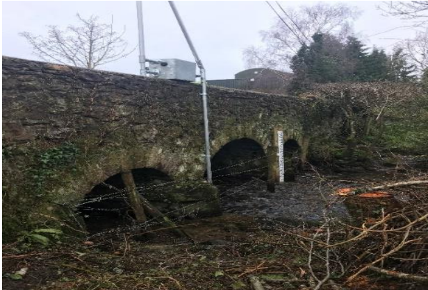
New Water Level Gauge – Coolroe
