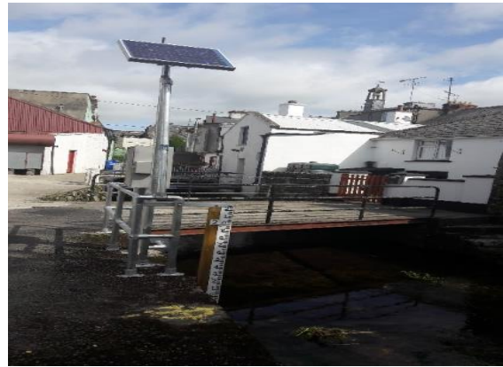
New Water Level Gauge – Turf Market
