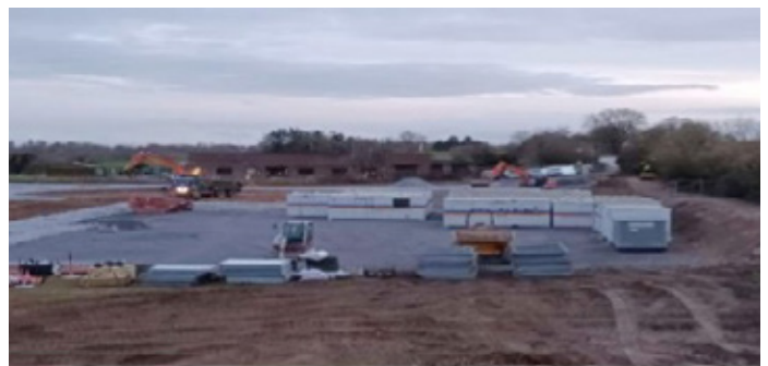
Compound setup including Safety, health and welfare facilities, offices, material storage and car parking
