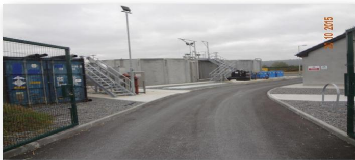
Freshford Waste Water Treatment Plant
