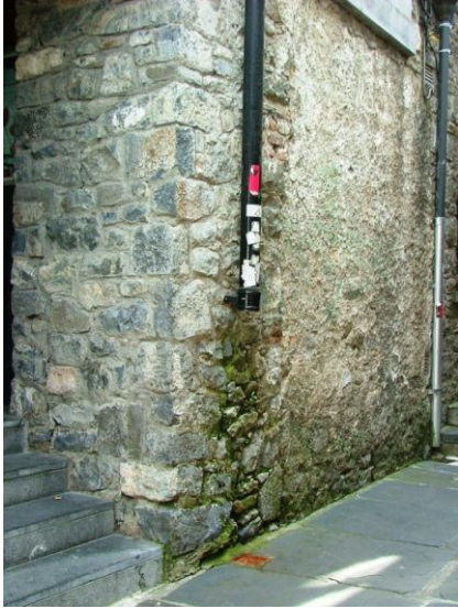
Example of rainwater downpipe failure.
