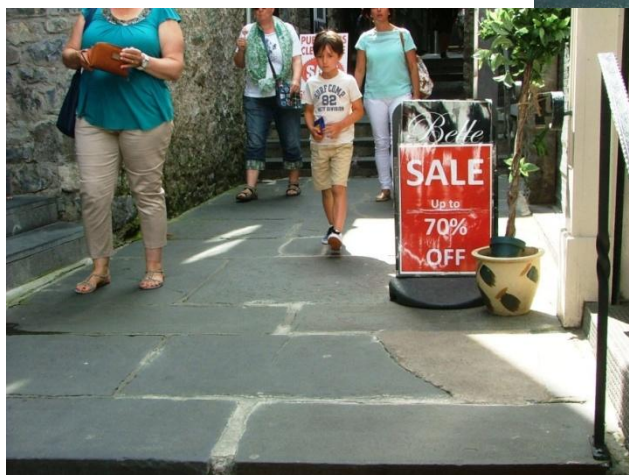
Pavement in middle of lane, at approach to lower steps.
