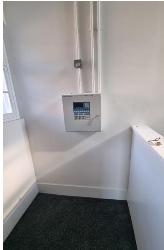
Fig.32 - Fire alarm panel
