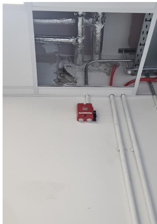
Fig 34. Fire stopping to escape routes
