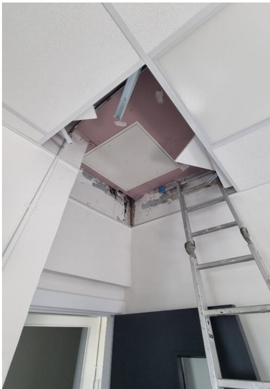
Fig. 33 - Fire rated access hatch
