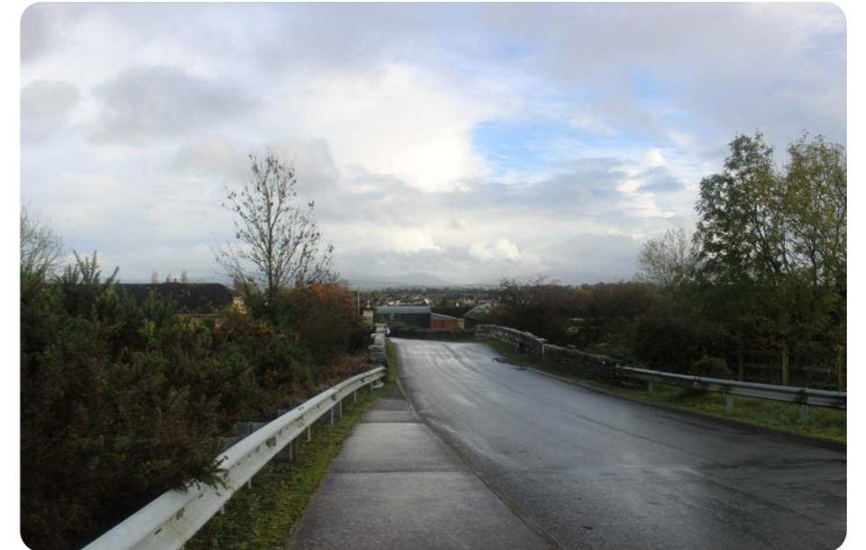
Figure 5.7: Footpath disappears along An Choill Rua
