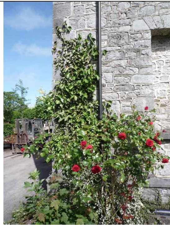
Fig.30: Ivy growth to the south elevation.
