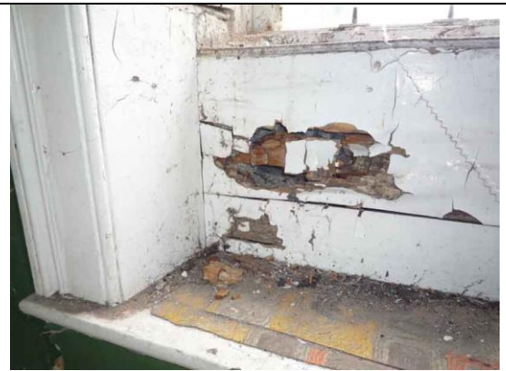
Fig.54: Timber decay of window back to west window opening of F11.
