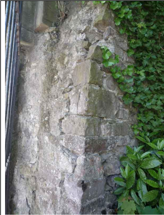
Fig.39: Pocket of destabilised masonry to a section of the southern boundary wall (adjacent entrance gateway).
