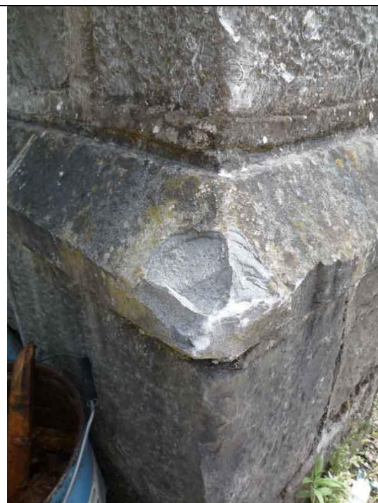
Fig.22: Chipping of stonework to the northwest corner of the south wing caused by vehicle impact.
