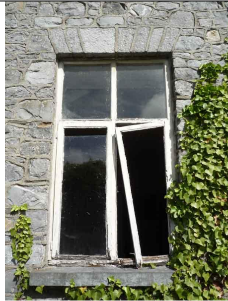
Fig.34: Complete failure of the timber casement windows.
