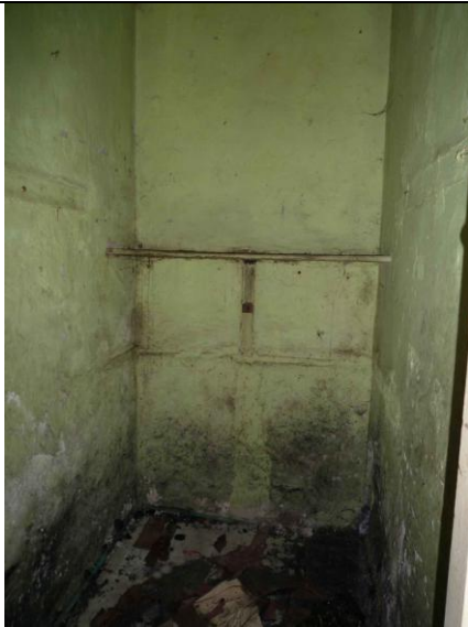
Fig.59: Plaster failure at low level as a result of rising damp to G20.
