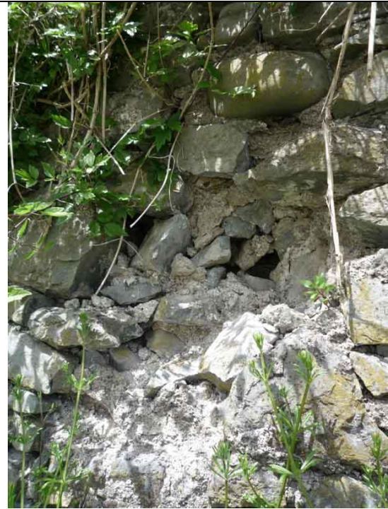
Fig.40: Pocket of missing and loose masonry to the northern boundary wall.
