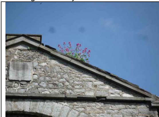
Fig.19: Scaling & detachment of stone to the horizontal string course to the south pedimented breakfront.
