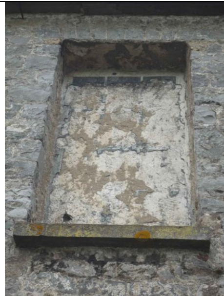
Fig.36: Blind window opening with trace remains of trompe-l'oeil window to first floor (east) of north elevation.
