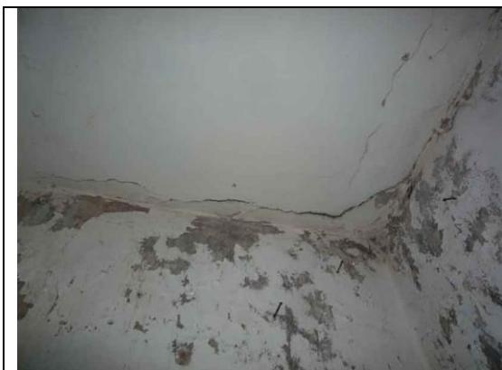
Fig.47: Cracking of ceiling plasterwork to G10.
