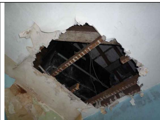
Fig.48: Significant hole in ceiling plaster over F01.
