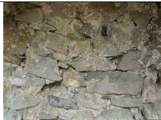
Fig.42: Open-joints to northern boundary wall.
