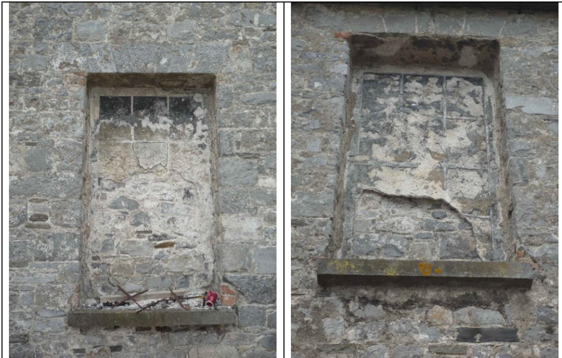
Fig.37: Blind window opening with trace remains of trompe-l'oeil window to ground floor (west) of north elevation.
