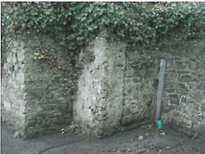
Plate 19. Untied walls at boundary at millrace.
