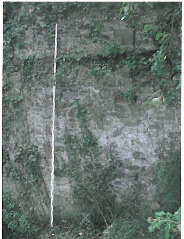
Plate 37. Internal end wall of building on Rocque, south west boundary. Scar of possible stairwell in wall.
