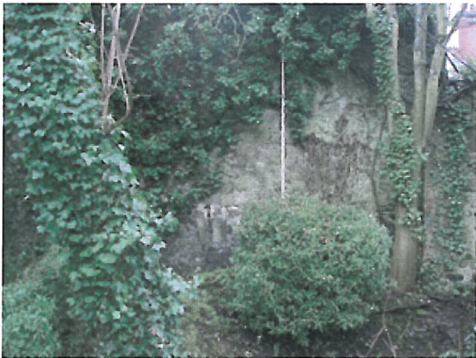
Plate 36. Scar of steeply pitched gable in plaster visible in western boundary wall.
