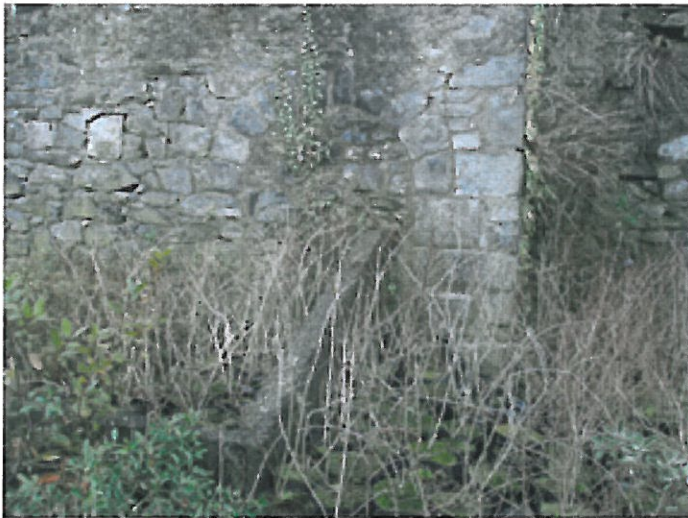
Plate 42. Round headed arch in late 18th or 19th century east site boundary wall.
