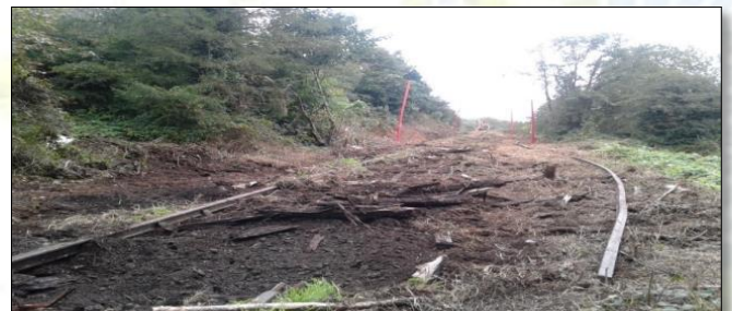
Lifting of old rails and sleepers along the route of the South East Greenway
