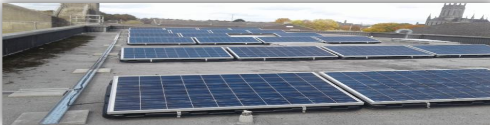
Kilkenny Fire Station 6kWp solar photovoltaic panels
