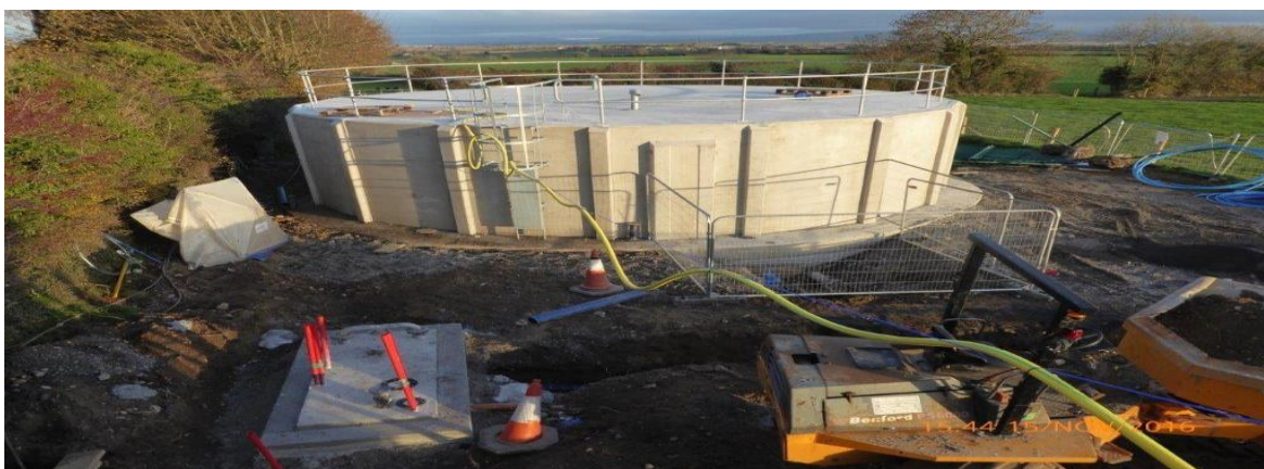
New Reservoir at Outrath
