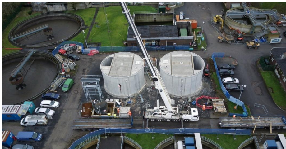
Sludge Import & Liquor Tank Installation Works – Kilkenny City & Environs Wastewater Treatment Plant
