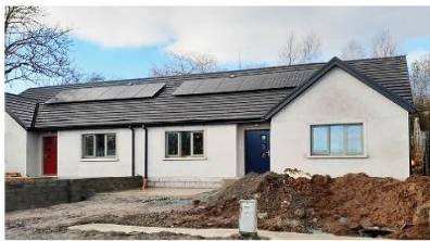
2 UNITS AT MULLINAVAT
