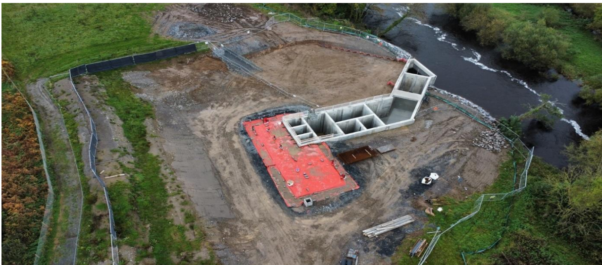
New Inlet Works – Kilkenny City RWSS Troyswood
