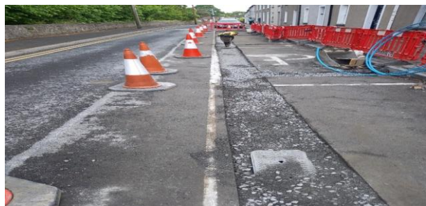
Transfer of services to new HDPE public-side mains at Michael Street, Kilkenny City
