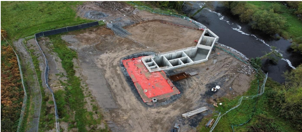
New Inlet Works – Kilkenny City RWSS Troyswood
