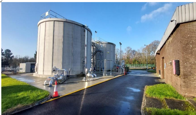
Kilkenny City & Environs Wastewater Treatment Plant Purcellsinch Completed Sludge Import & Tank Installation Works
