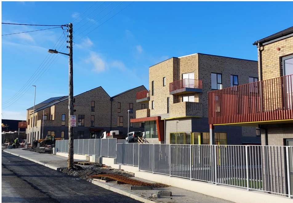
Completion works ongoing at Crokera Hill, Kennyswell Road – 88 unit and community centre
