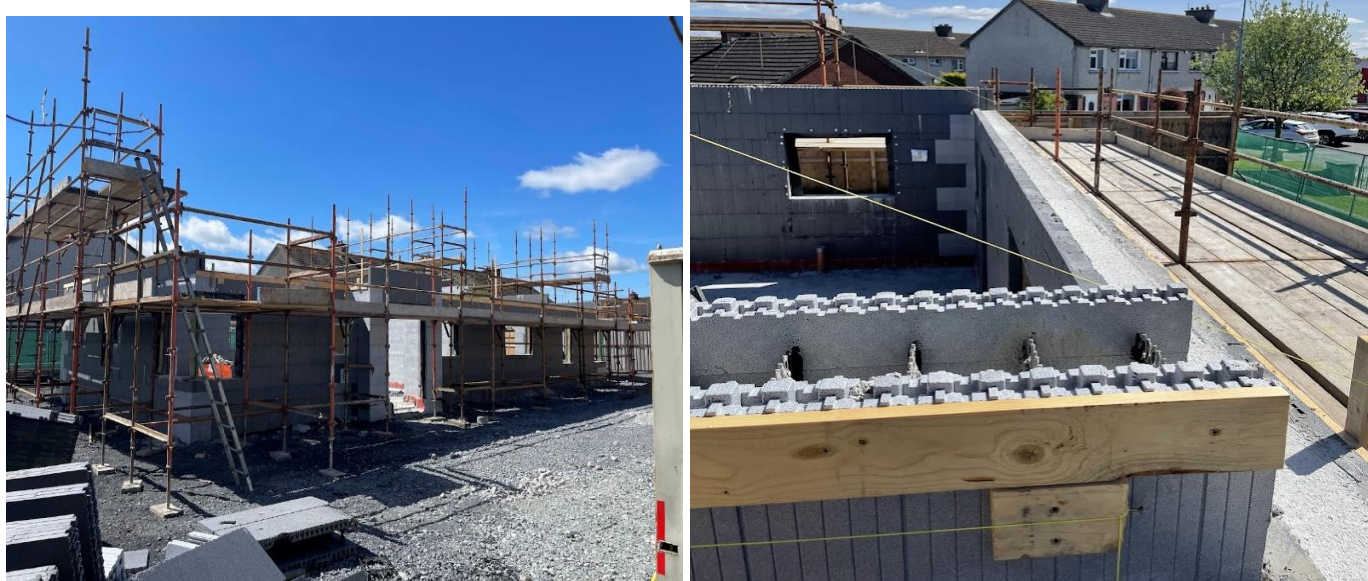
Construction of 2 Wheelchair Accessible Houses at the Old Community Center in Loughboy, Kilkenny The Houses are being constructed using Insulated Concrete Form (ICF)
