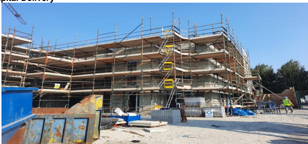
Turnkey Housing Project - 22 Social Housing Units under construction on the Callan Road / Cicular Road Junction. Estate to be known as "Marnellsmeadows" to reflect the history of the townland. 4 x 2 bed units, 9 x 1 bed and 9 x 3 bed.
