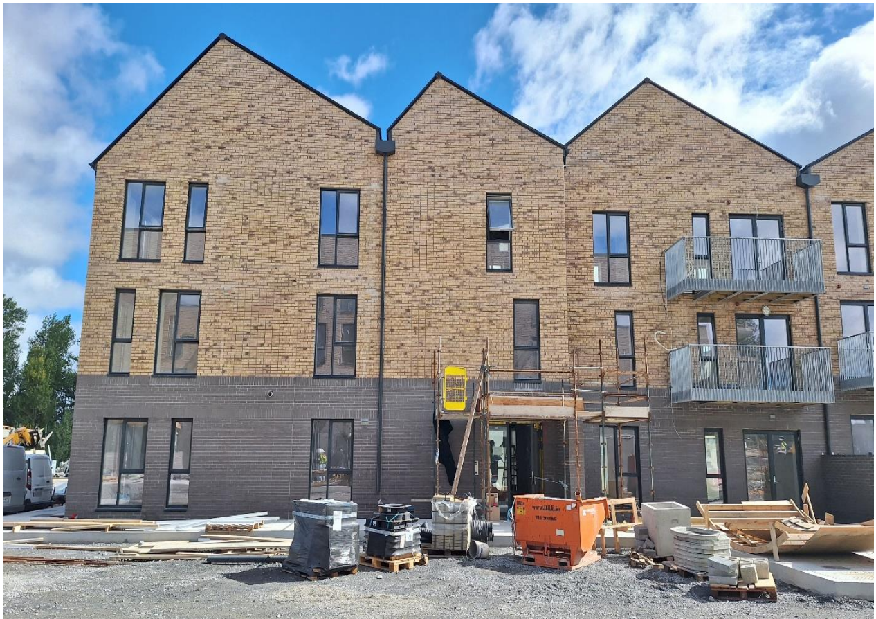
Direct Build Housing Project progressing on site – 88 units + Community Centre at Crokers Hill, Kennyswell Road, Kilkenny City
